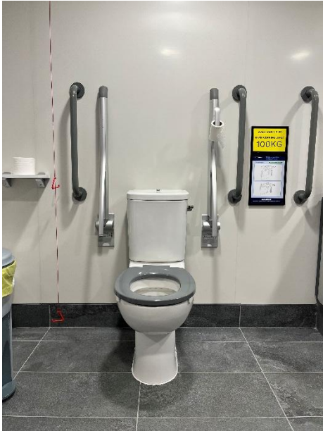
Toilet with pull down handles. Red emergency cord to left of the toilet.
